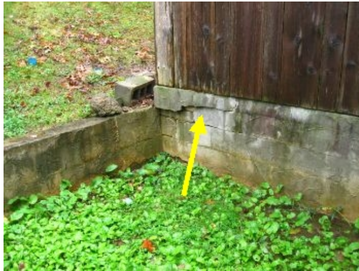
wall is falling in.
