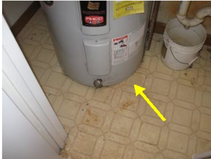
water heater is missing the water heater pan
